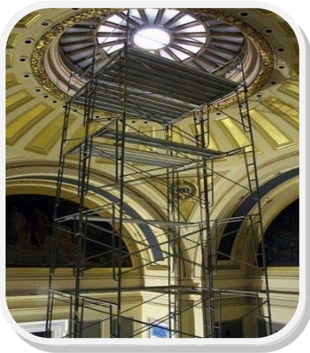
The State Capitol renovation included removing coverings from the courtroom's skylight. (Minnesota State Capitol Restoration photo. More photos available at https://www.flickr.com/photos/capitol-restoration/ .)
